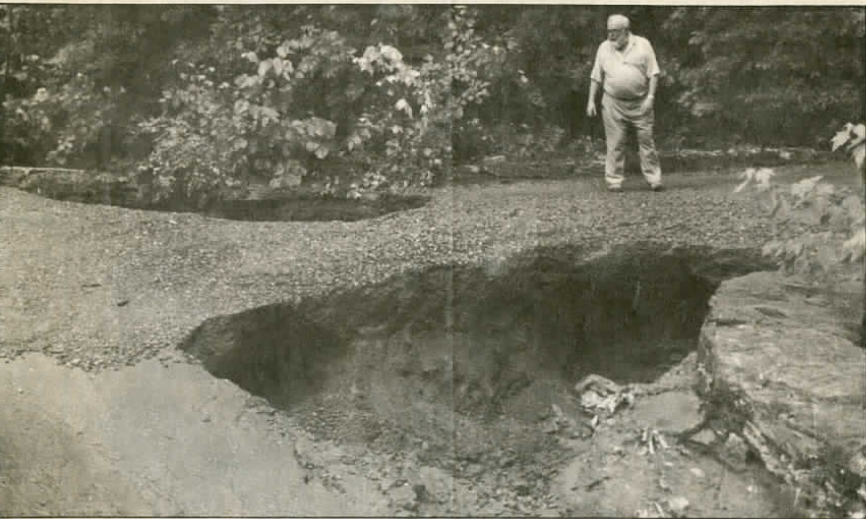
HOLY MOLEY — George Rublee of Cornish stands on what's left of Platt Road in Cornish on Sunday, observing the handiwork of Mother Nature. Local police and highway crews reported mostly minor washouts and power outages caused
