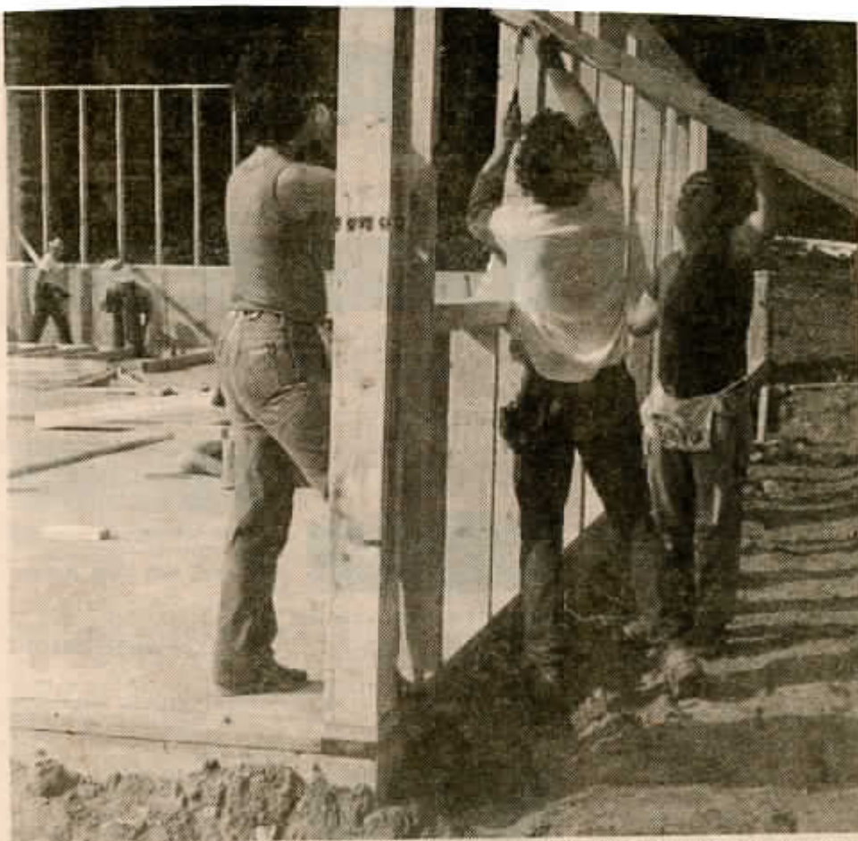
FIRE STATION CONSTRUCTION— While one volunteer, left, takes a cold drink, two others attach a support during the construction of the Cornish Fire Station June 9-10. (Ruth Rollins Photo)
