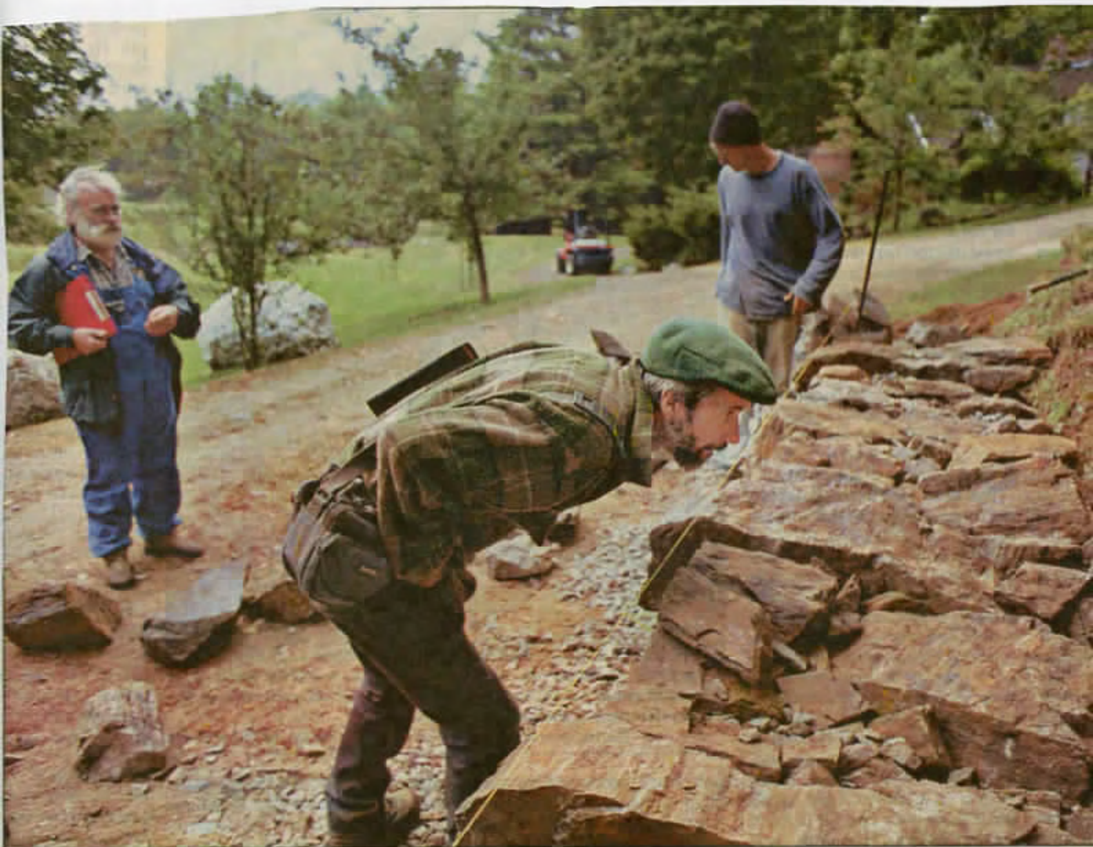
Bruce Curtis, an examiner with the Dry Stone Walling Association of Great Britain, gets a close look at a retaining wall being built by Travis Callahan of Claremont (background). Fellow examiner Dave Goulder is at left. Callahan
