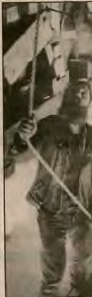
JOHN FERLAND, a foreman for Chesterfield Associates, moves some beams of the trolley running the length of the Cornish-Windsor Covered Bridge. (Julian P. Brown Photo)
