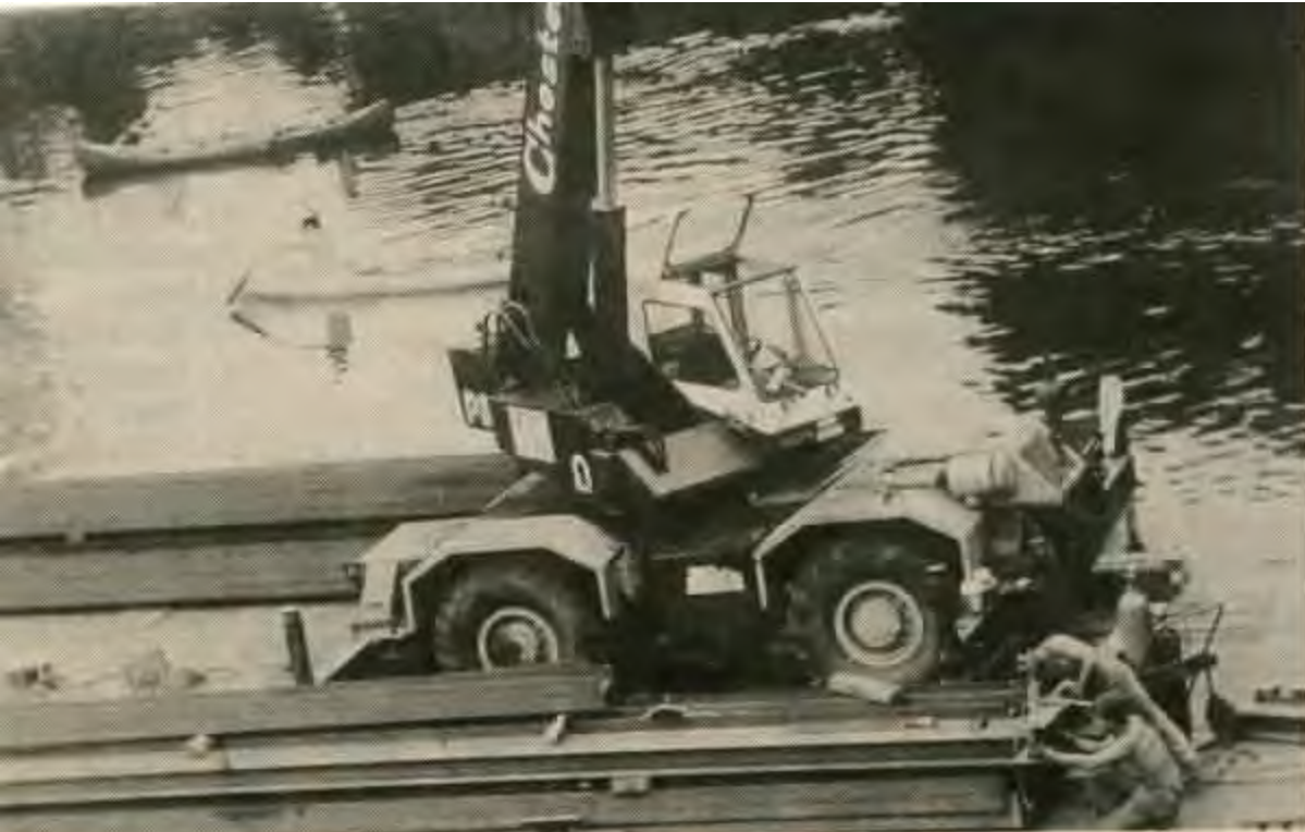
WATCHING THE RIVER FLOW -- Two canoes pass by the barge and crane being used by Chesterfield Associates in its restoration work on the Cornish-
