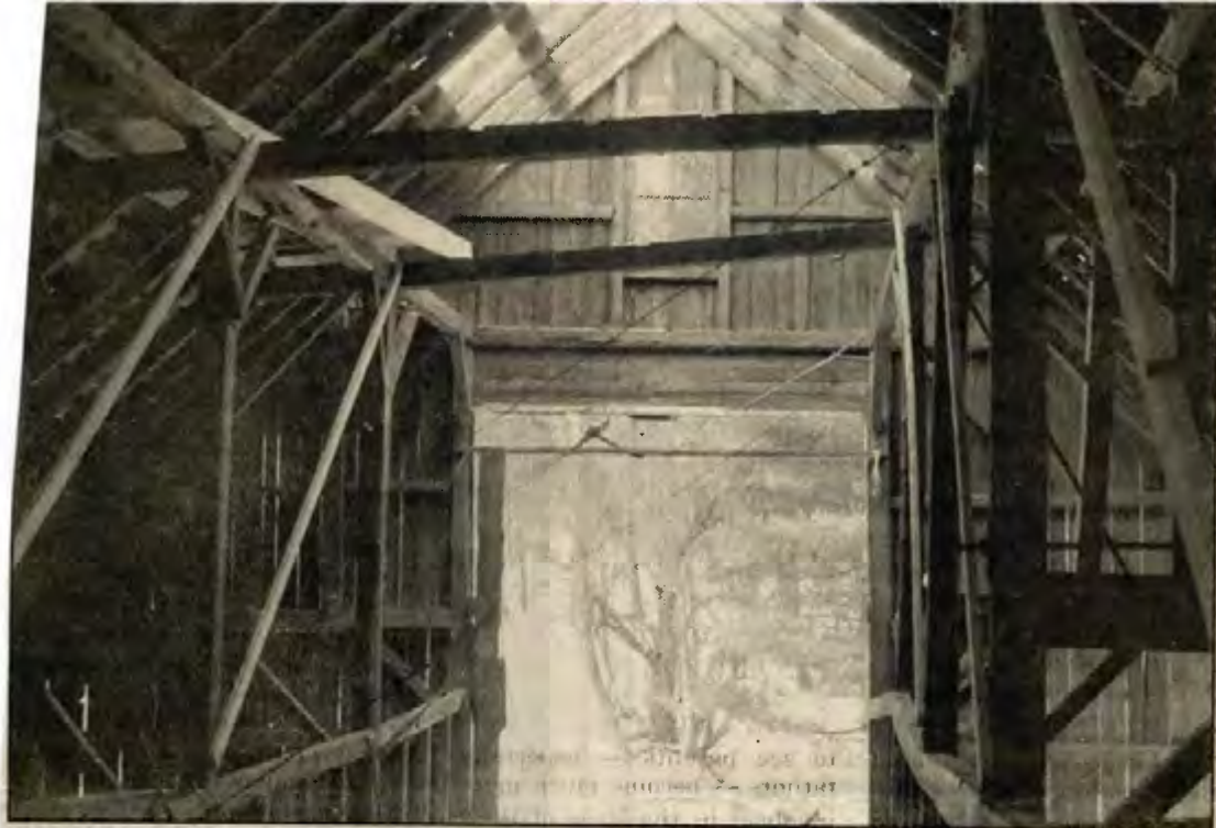
COMING DOWN — This barn is being dismantled and moved from Newport to Cornish (Christian Berkey photo)
