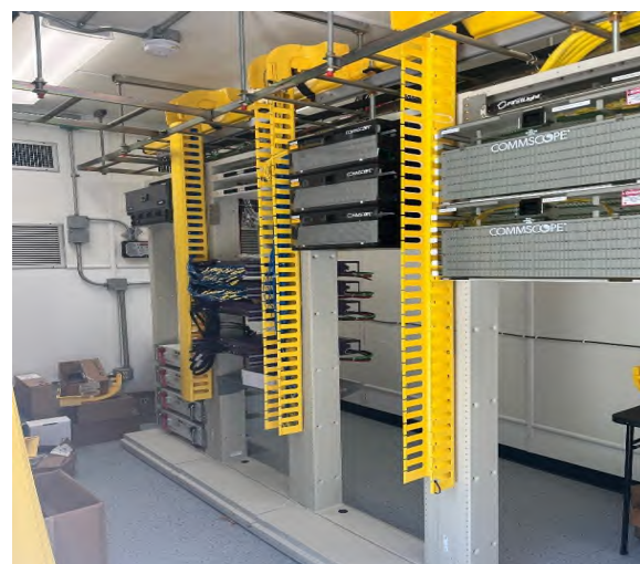
The Fiber Electronics Hut in Sandwich
