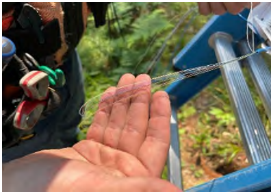
Splicing a fiber strand in Sandwich to make it ready for customer drops
