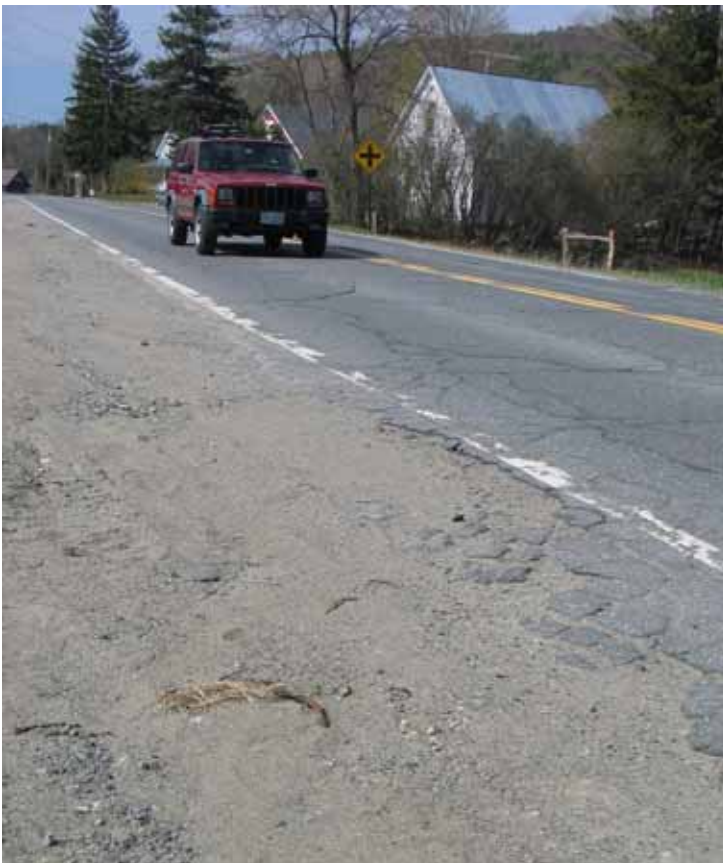
Deteriorated pavement conditions on Route 120 in Cornish Flat.
