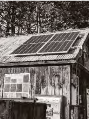
Solar at Cornish Recycling
